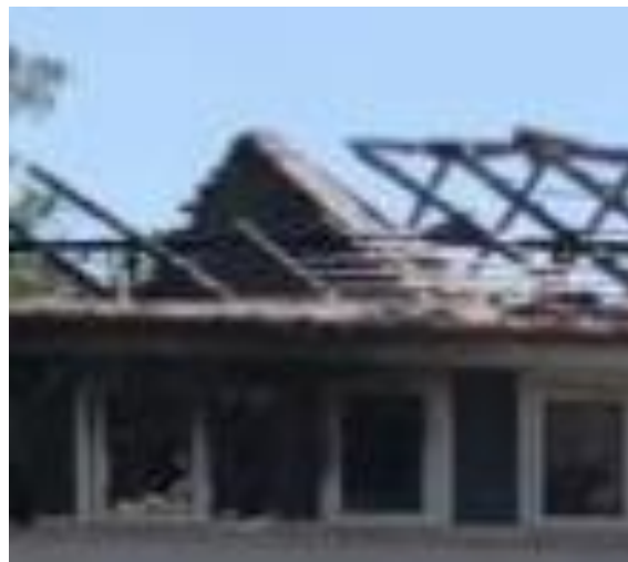
6. An enlargement of part of the previous photograph showing the party wall between no 11 and no 13. Most of the tiling battens have been destroyed by fire but some remain in place near the eaves. There should have been fire-stopping between the battens where they pass over the party wall: none is visible. It might have fallen away in the fire but I think it more likely that it was never present.
