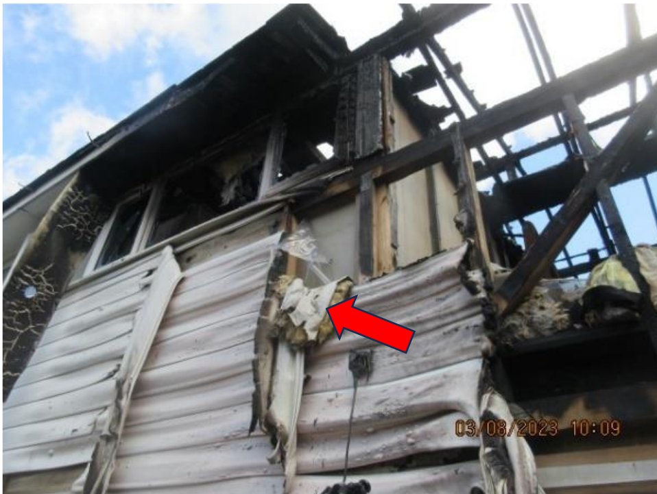
12. At the rear of 13. Some uPVC cladding had been softened by heat and had fallen away, exposing the wall frame behind. There is no underlying plywood at this point just mineral fibre (arrow) and the plasterboard inner lining. There has clearly been no spread of fire over the cladding here.
