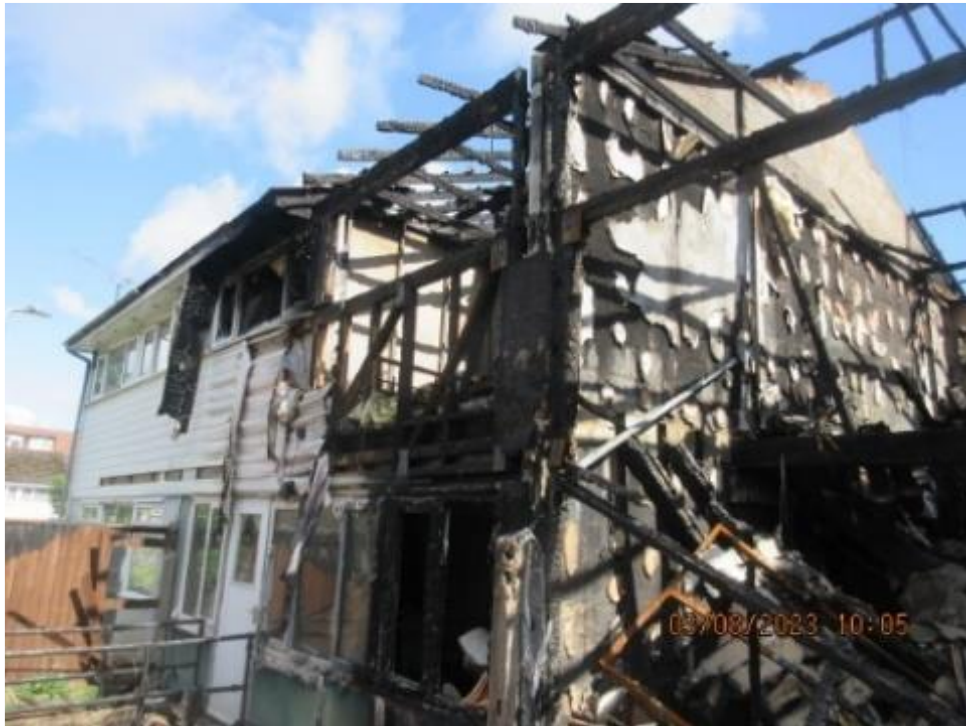
7. At the rear. A blackened section of uPVC eaves soffit is hanging down at the approximate position of the party wall between 15 and 13.
