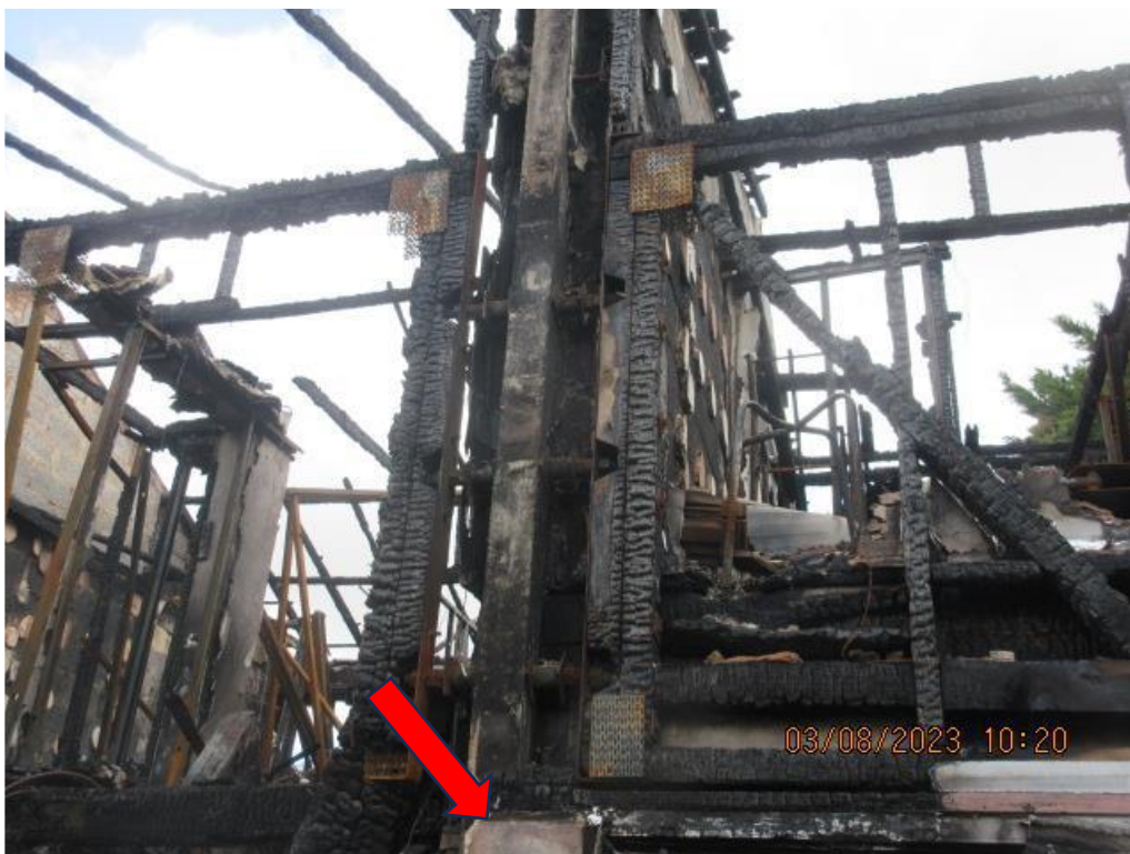
13. The party wall between 11 and 9. The wall frames of each house had been bolted to a concrete support post with the party wall built tight against the back of this post. The spaces between the post and the edges of the wall frames had presumably been packed with insulation and covered externally by some board material, now destroyed. A section of what appears to be a non-combustible board remains in position (arrow). This might have been a later repair given that it is only present on one side of the party line.
