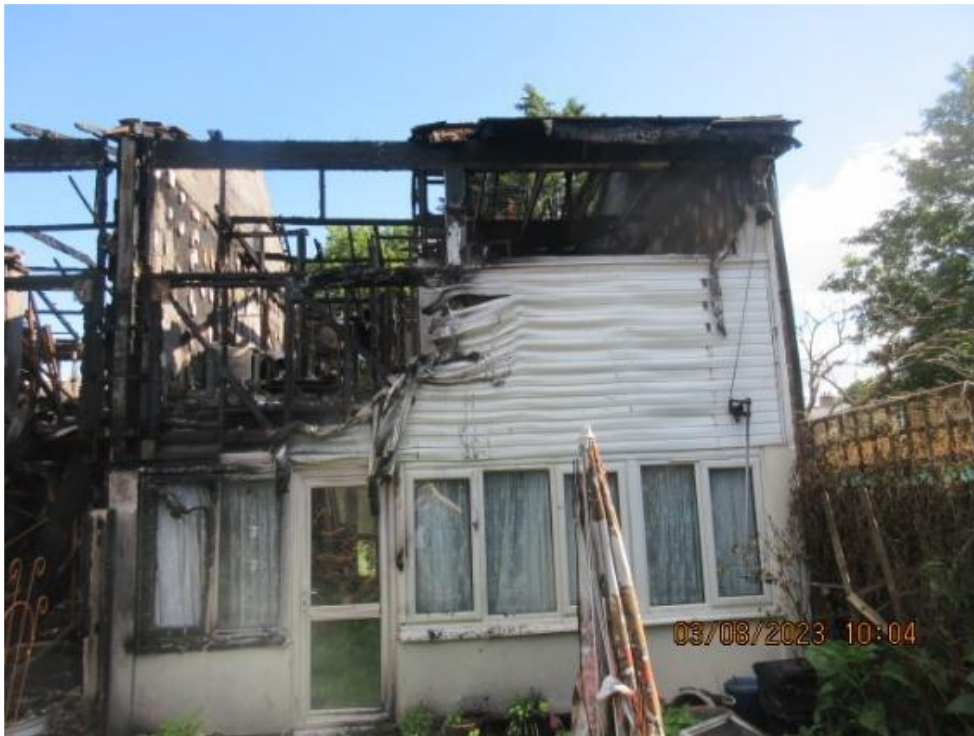
11. The rear of no 9. The destruction of the uPVC cladding seems to have been caused partly by direct flame impingement from the external fire involving the yard of 11 and the intervening fence, and partly as a result of fire inside the house burning through the plasterboard on the inside of the wall frames. The cladding remaining in place is damaged by heat but there has been no spread of flame across its surface.
