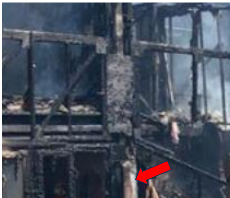
14. An enlargement of part of photograph 8 showing a charred area of board covering the concrete support post between 13 and 11. This could have been plywood. It would have been covered by the uPVC cladding. I doubt that there could have been a cavity allowing horizontal fire-spread behind the board and I also doubt that there would have been much of a gap between the board and the uPVC cladding. The arrow indicates what appears to be a section of non-combustible board half the width of the charred board.
