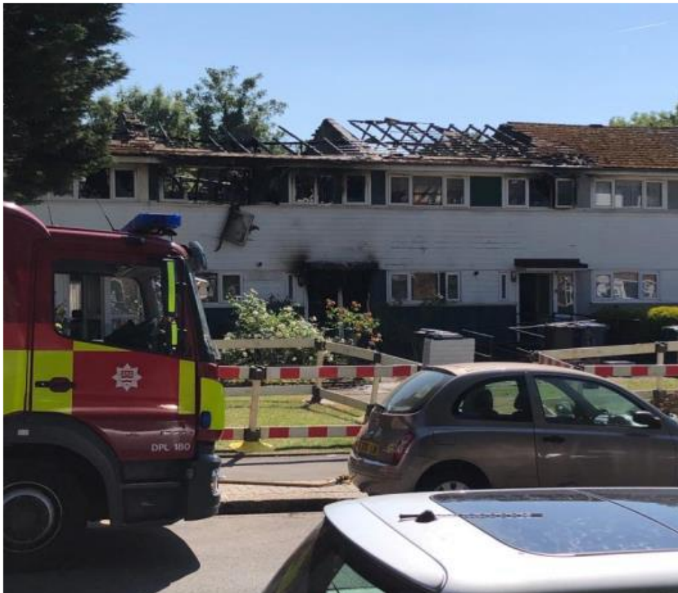
5. The front of the terrace. No 9 is on the left, mostly out of view. The house with the most severe damage is no 11, with 13 at centre right and 15 on the far right
