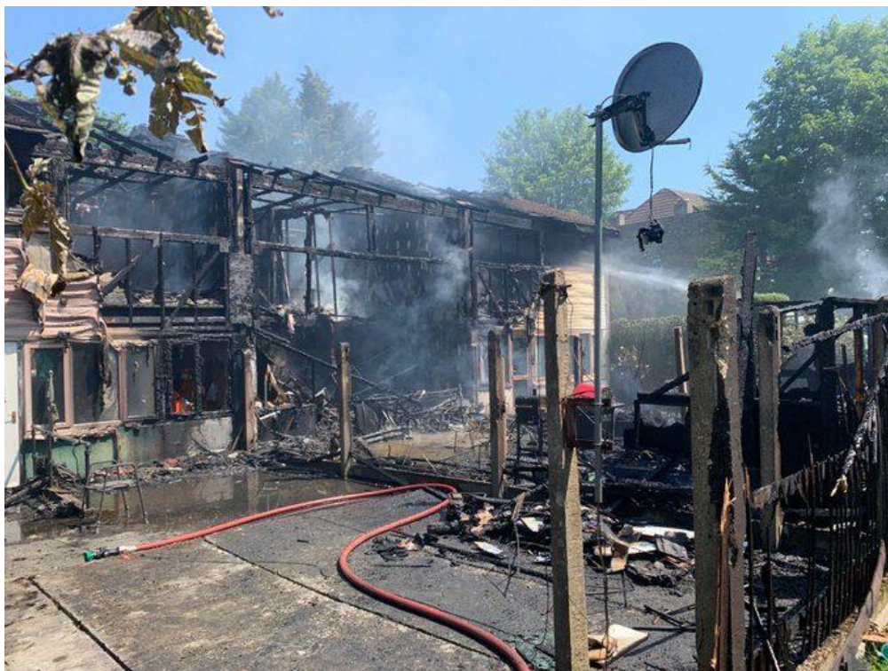
8. The yards at the rear of 13 and 11 seen from beyond the line of the rear fence. The pattern of damage to the uPVC cladding corresponds to what I would expect from flames from a severe fire burning close to the building and involving the whole width of the yard to no 11, plus the fences on either side. This flame impingement seems to have extended beyond the lines of the party walls to destroy areas of cladding on both no 13 and no 9. This photograph, copied from Parikiaki, was taken by the London Fire Brigade.
