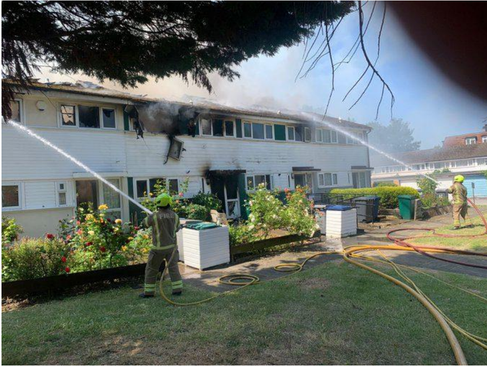
The front of the houses. No 9 is on the left. No 15, the least damaged, is at the right-hand end of the terrace. Note that there has been no fire-spread across the uPVC cladding visible at the front of the terrace, despite severe fire conditions within the centre two houses seen in this view.
